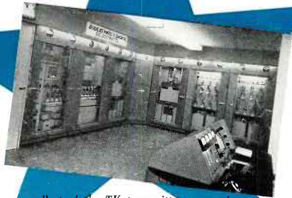
Part of the TV transmitter room of WLW-A, Atlanta, Georgia, an SE BLUE STAR STATION, showing visual end of Crosley Broadcasting Company's new 50 KW transmitter, 316 KW ERP. 100% air cooled.
