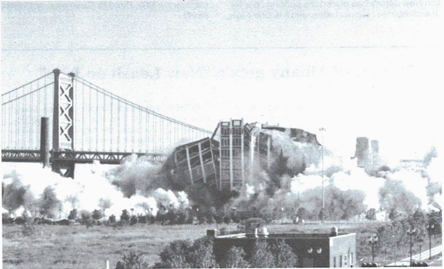
Figure 4. Two RCA buildings along Camden's waterfront are demolished in a few seconds at 8 A.M. on
