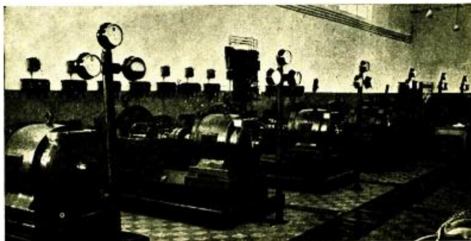
Power room of the Comintern Station, at Moscow. Note that the meters are mounted on stanchions.
