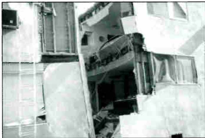
A condemned apartment building in L.A.'s Sherman Oaks area, where the effects of the quake were particularly intense, continues to crumble under its own weight.
