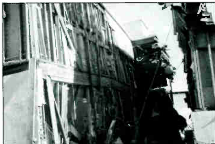
Another Sherman Oaks building sheared in two by the quake.
