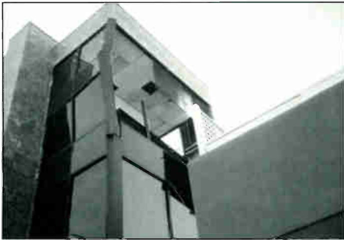
Buildings were twisted into pretzel-like shapes by the force of the temblor.
