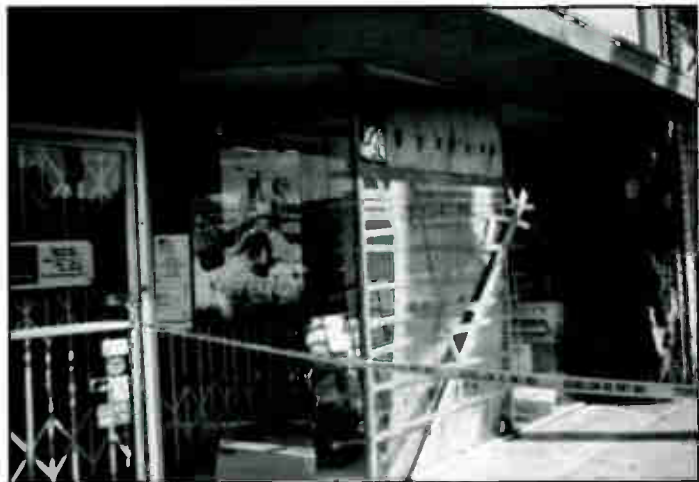
For Tower/Westwood's Rick Dorsey, it was like "someone picked up the store, turned it upside down and dropped it."
