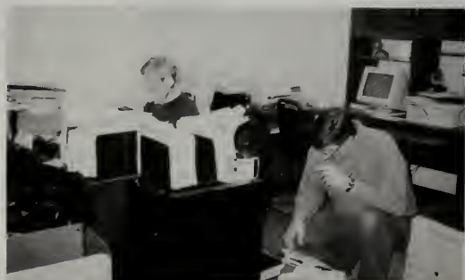
Meanwhile, back in Chicago headquarters, Carol and Rus Strahan (l-r) are managing to conduct "business as usual" while extensive renovation and reconstruction is in progress.
