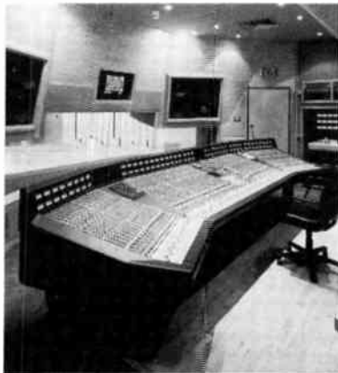
The new Solid State Logic 72-channel 4000 G Plus board, at Town House's Studio One, happens to be the U.K. manufacturer's 1,000th console installation.
