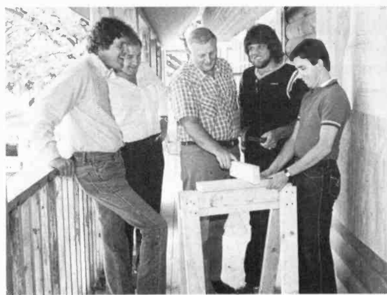
CONTRACT CONSTRUCTION —Artist Marlow Tackett, second from right, celebrates his signing to RCA Records, Nashville by assisting in the construction of the new site of Music Mill Studio owned by Tackett's producer Harold Shedd. Locking on from left are: Shedd; Donny Canada, Tackett's manager; Jerry Bradley, division vice president, RCA Records, Nashville operation; Tackett and Joe Galante, division vice president, marketing, RCA Records, Nashville.
