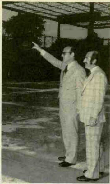
PIONEER EXPANSION —Contractor Charles Klatskin, left, points out progress on 43,000 square foot branch addition to Bernie Mitchell, U.S. Pioneer Electronic President. With completion in November, the Moonachie, N.J., warehouse/quality control/sales/service facility will have 125,000 total square feet.
