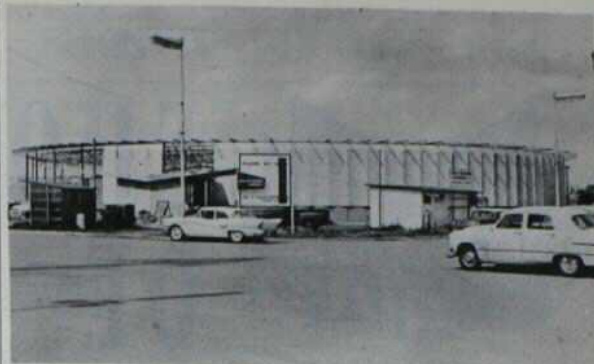
The '59 Oklahoma State Fair, Oklahoma City, will offer fairgoers another new feature, a new Art Center, shown above in an advanced construction stage. The ring-shaped building, which will have an inner circle of 99-foot diameter for an outdoor exhibit area, will cost $300,000.
