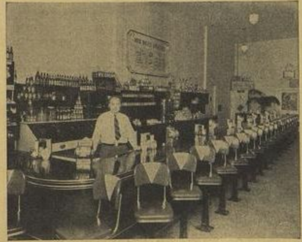
PACKARD PLA-MON REMOTE-CONTROL INSTALLATION in the United Waflag Shop, Houston, Tex. The installation was made by the R. & A. Musto Company, Houston, which reports receipts have jumped since the equipment was put into use.
