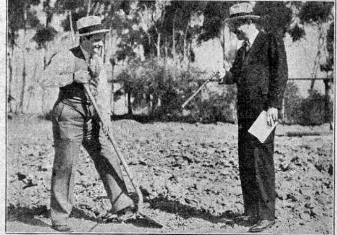
NO SOONER had Lew Dufour and Joe Rogers arrived on the lot of the California Pacific International Exposition, San Diego, Calif., than Lew suggested that Joe whip off his coat and break ground. "This is as it usually is," Joe remarked as he bent his back over the shovel, while Lew laughingly directed operations with that new cane he brought back from Paris.
