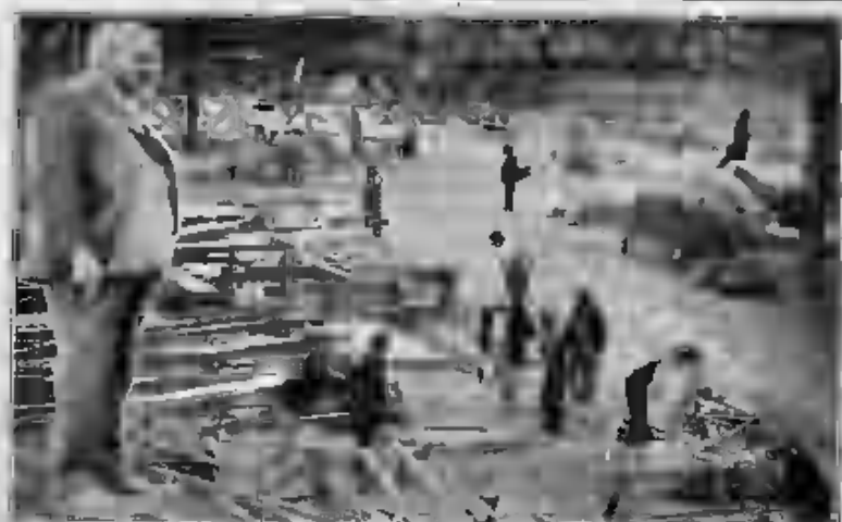
P. T. STRIEDER, genial general manager of the Florida Fair, Tampa, looks over activities on the grounds where buildings have been wrecked to permit a rebuilding and expansion program in which $228,000 will be spent on improvements.
