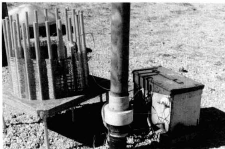
Photo C. Power amplifier, base insulator, and loading coil at the base of the transmitting tower. The coil is about 100 turns of 28/10 litz wire. About 75 turns are being used at present. A 50" × 50" mat of chicken wire lies just below the gravel. The tower is 50' high.
