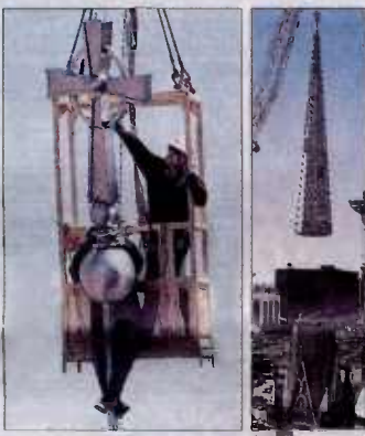
At left, Jerry Holt, standing, and Marty Dickerson accomplish the tough job of threading an 8-foot-8-inch-tall, stainless-steel Celtic cross into a mast atop the new Old Stone Church steeple on Public Square. An aluminum replica of the original spire, right, is moved into place atop a steel base anchored to the church. The men made two ascents to 200 feet before managing to maneuver the 300-pound cross into place amid 22 mph winds. For a detailed look, see tomorrow's religion section.
