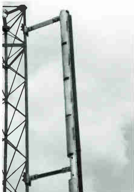
One of the Dielectric Communications LPTV antennas.
