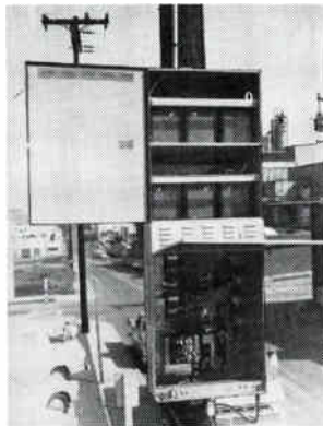
MODEL 1150: Single, self contained module including battery compartment: 900VA. MODEL 1042: Compact cabinet design (38" high) includes 3-battery compartment: 720VA.
