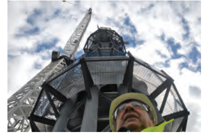
Lyons standing beneath the erected spire and lighting rod atop One WTC.
