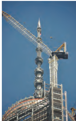
The new spire is erected added to the top of One WTC.
