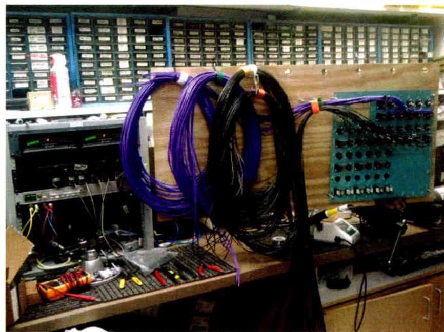
Key to the Soundbite truck is its main I/O panel, seen here as it was being wired.
