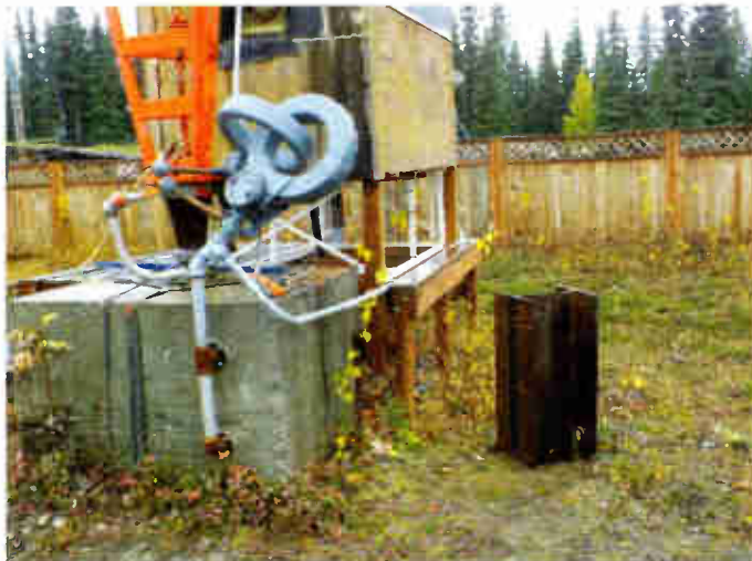
One of the completed pilings by the base of the existing tower. It will be used as part of the foundation for the replacement tower.
