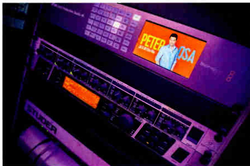
The Blackmagic Design ATEM camera controller tops the rack equipment.
