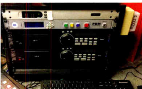
The Telos Hx1 hybrid provides the phone interface for the mixer at WDNP(LP).
