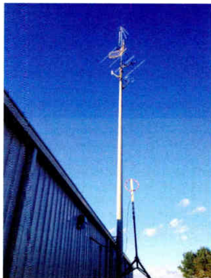
Fig. 2: STL, two-way, FM monitor and EAS antennas are mounted to the pole.
