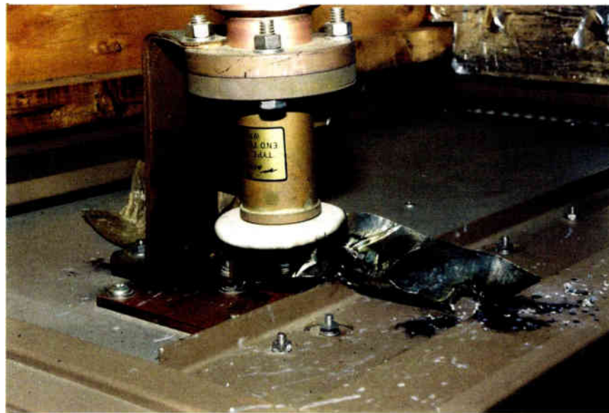
Fig. 1: Insulating foil tape fell down and shorted the transmitter output.
