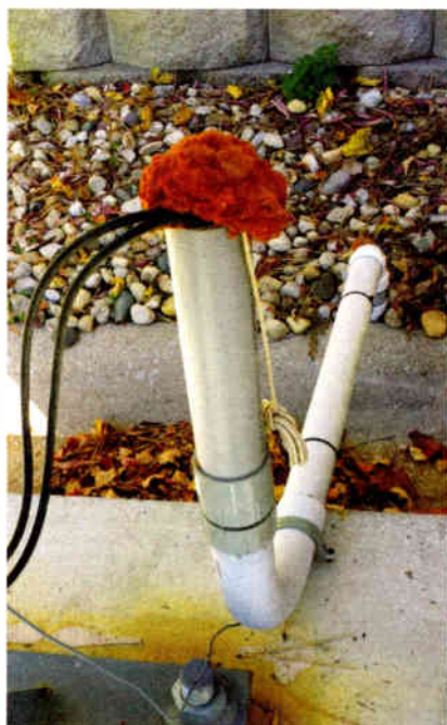
Fig. 2: With spring approaching, check all conduit openings and seal holes with expanding foam.
