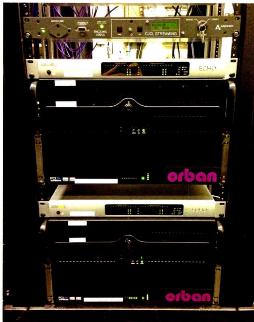
A pair of easily identified Orban OptiEXP expansion chassis at the Rogers Broadcasting Toronto facility.
