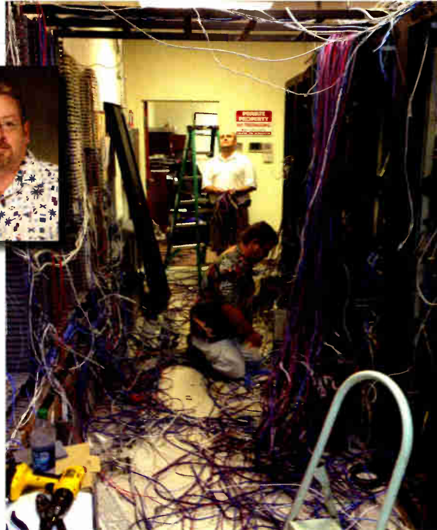
Charlie McCoy, inset, also is shown working knee-deep in wiring pulling out old cable. Standing is Dave Cooke, IT manager in Fayetteville.
