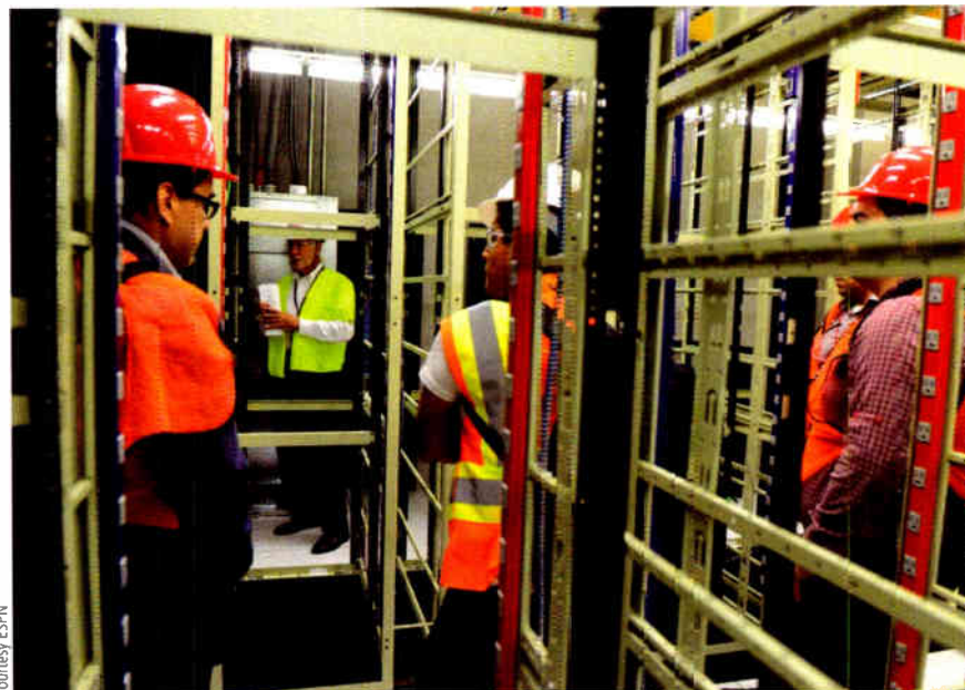
ESPN Vice President of Technology Planning Jim Servies, in yellow vest and seen through rows of waiting racks, conducts a construction tour of facilities in Bristol, Conn. He will speak about audio considerations of the project at the AES show in New York.
