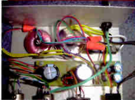
The guts of the power supply inside the box.
