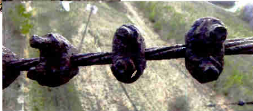
Fig. 2: Tower inspections can also uncover things like rusted cable clamps.
