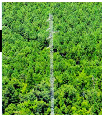
Aerial view of the WKMH(FM) Shively Log Periodic Directional FM Antenna in service.
