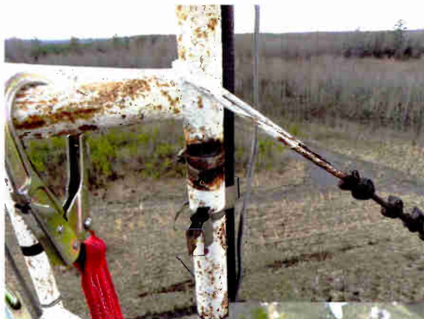
Fig. 1: A bullet pierced a leg of a tower; the damage was noticed by a tower rigger performing a quarterly inspection.
