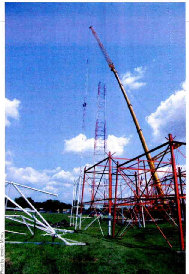
Glen Clark is one of the consultants commenting in this article. Asked for photos of AM projects, he shared this. Clark created an upgraded antenna design for Disney-owned WMVP(AM), Chicago in 2006. New antennas replaced a legacy three-tower array dating to the 1940s.
