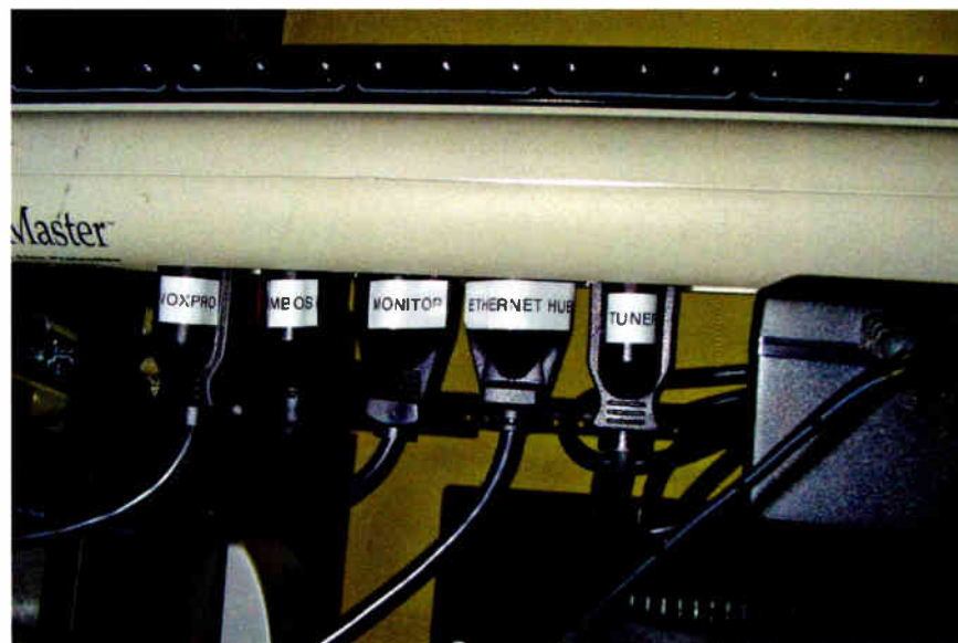
Fig. 2: Label plugs at the outlet strip to speed troubleshooting and identification.
