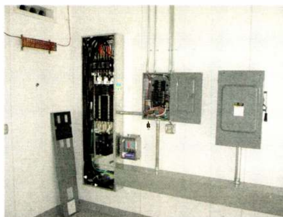
The electrical system comes pre-configured to the customer's specifications, in this case a three-phase disconnect for a 30 kW FM transmitter.
