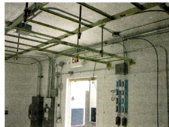
Cable ladders, 'halo' ground, telco board and high/low temp alarm thermostats are available options.
