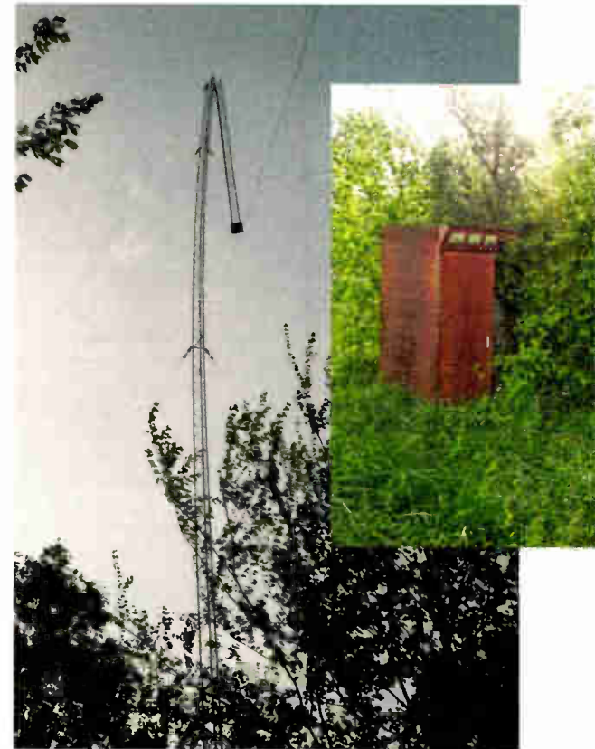
Fig. 2: Mother Nature takes a swipe at an AM tower. The top section eventually broke free.
