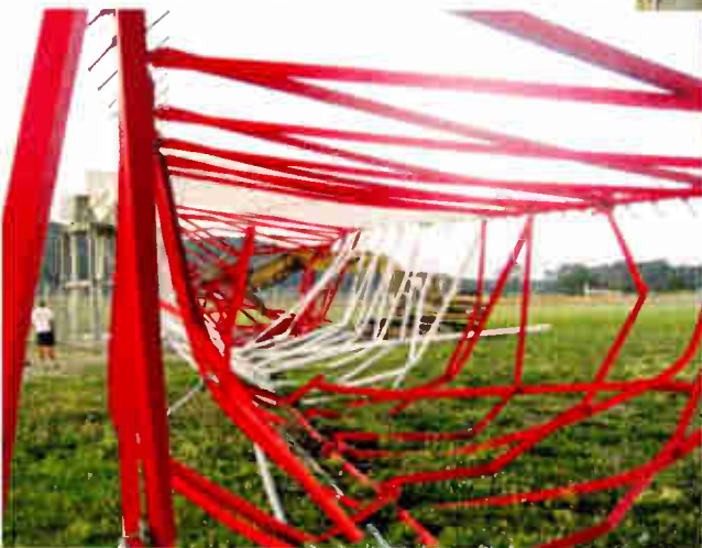
The track hoe used to damage the antenna system is visible through the fallen steel. The vehicle had been stored behind a locked fence made of anti-climb wire and stranded with barbed and razor wire.
