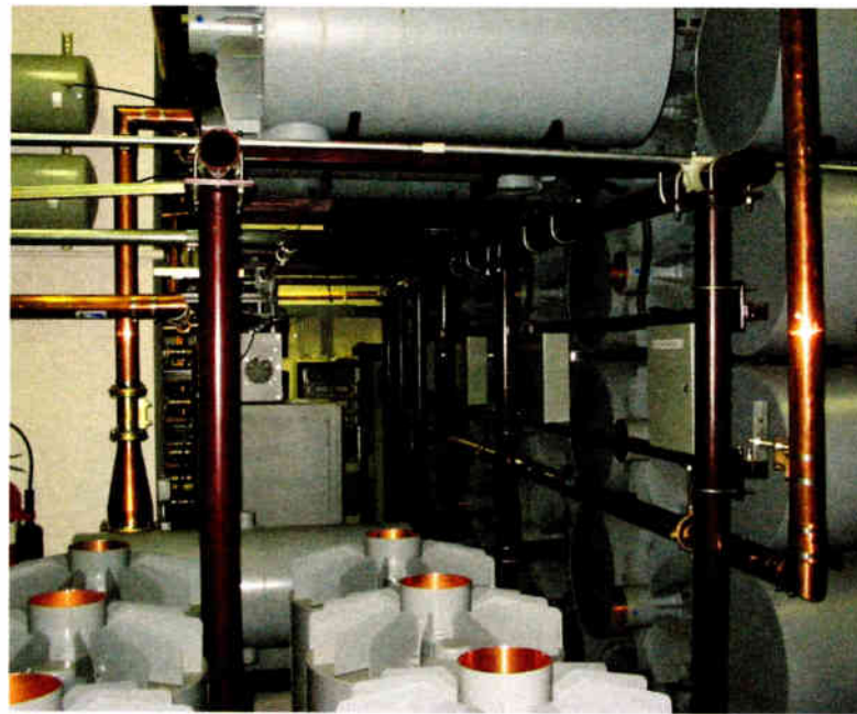
The center aisle in Empire's Master FM room.
