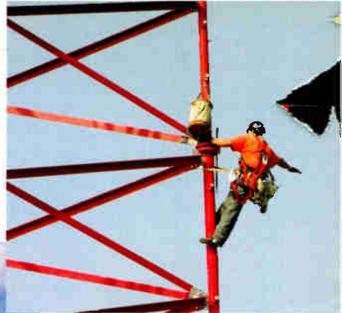
Jason Kardokus, owner of NorthStar Broadcast Contractors in Seattle, calls ‘Stop’ during the reconstruction.
