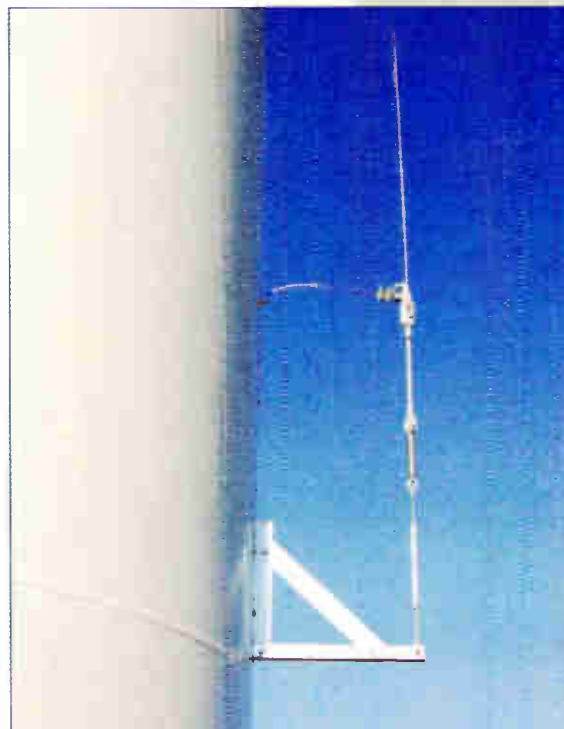
The wind tower's pedestal was factory modified to accept unipole hardware from Nott Ltd.
