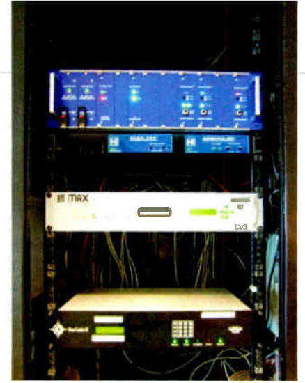
APT Oslo tops the rack.
