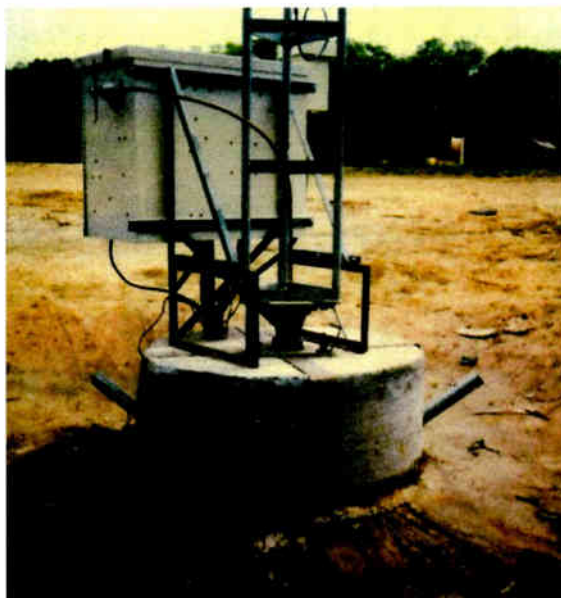
Fig. 1: A new tower site, but can you spot the problems?
