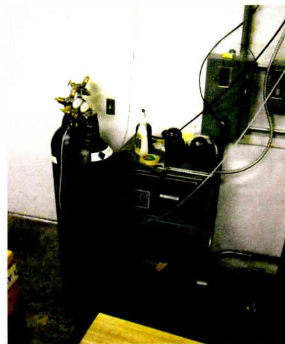
Fig. 2: Note the spiral wrapped cable coming from the box.
