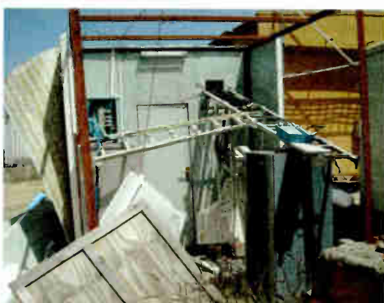
Fig. 4: It's a miracle the buildings were spared, beyond coax being yanked through the walls.
