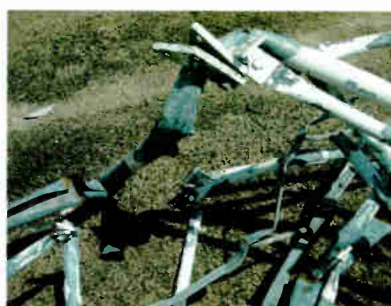
Fig. 5: Tower section flange bolts popped, offering an idea of the forces involved.
