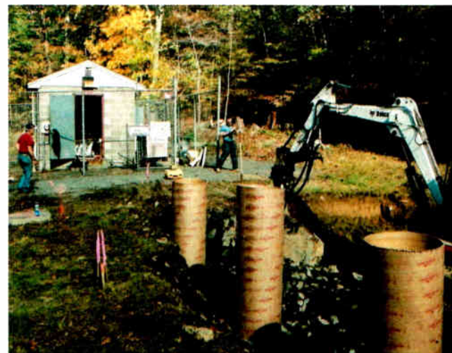
The construction crew has installed the first row of tubes for pouring concrete piers to create a level base for a pre-cast concrete transmitter building. The vertical rebar in the tubes actually is attached to the ledge via grouted holes.
