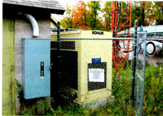
At the main WXPR transmitter site on Thunder Lake Road in the town of Sugar Camp, Oneida County, Wis.
