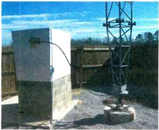
High-Power Antenna Tuning Units
