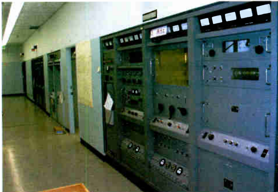
One of the three hallways in the 'transmitter horseshoe' at WWV. Each of the frequencies has a main and backup transmitter. Main transmitters are modified CCA transmitters, backups are Technical Materiel Corp. Each frequency is auto switched to its backup in the event of failure of the main.
