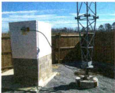
High-Power Antenna Tuning Units
