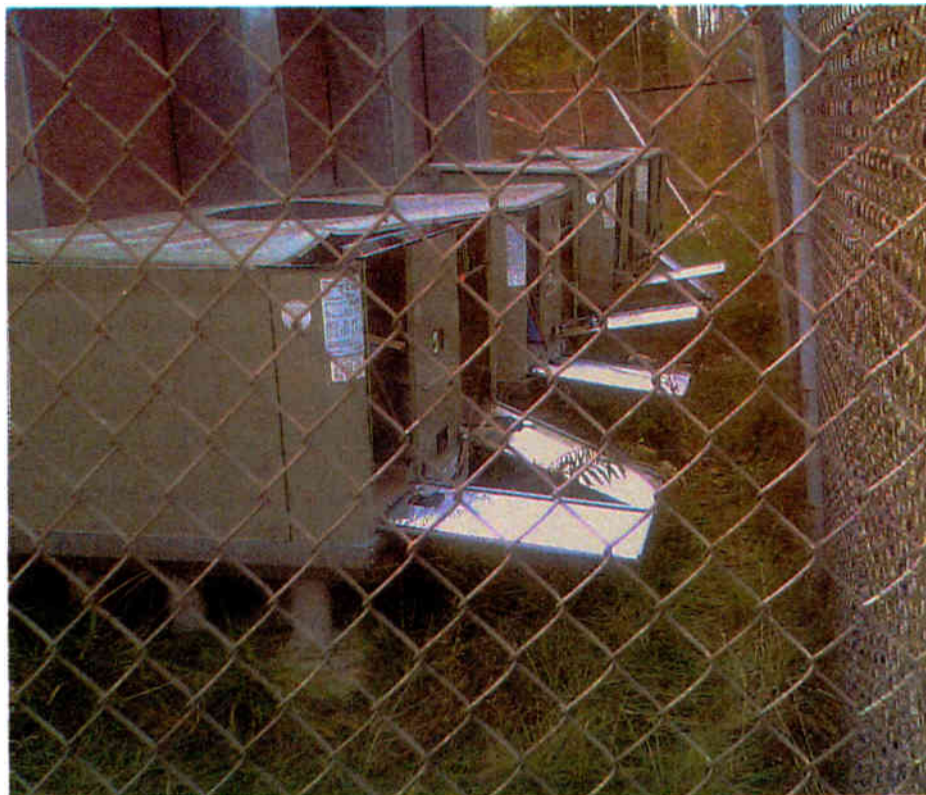
Cumulus' Indianapolis cluster had their air conditioners broken open with condenser and evaporator coils stolen.
