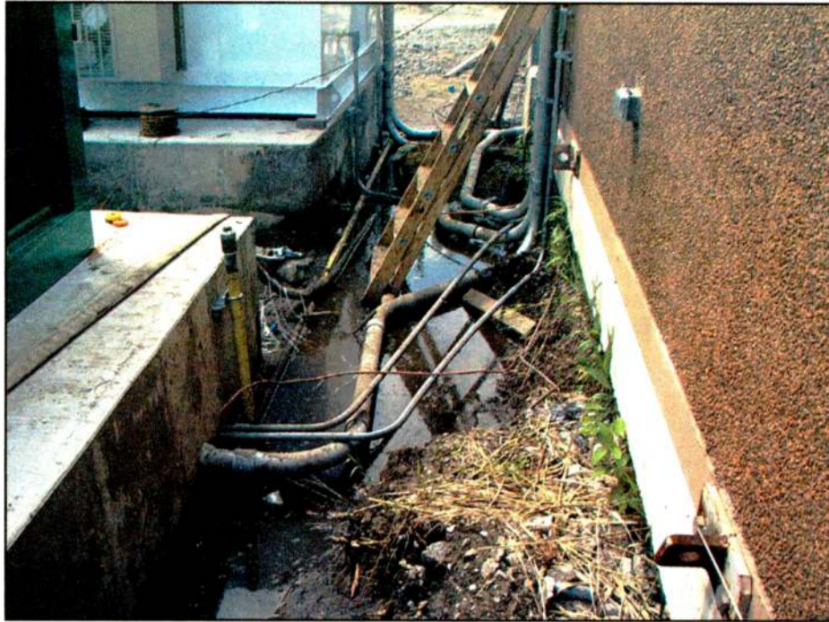
Fig. 2: This was the area of greatest concentration of wiring. Pictorial documentation of such a project is vital to prevent future accidents due to digging at the site.
