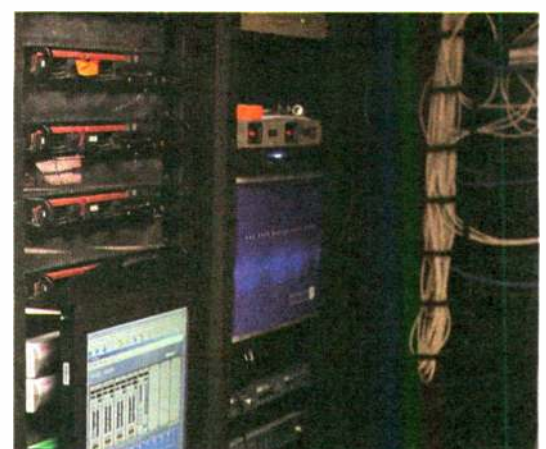
Pictured is our installation in the New York studios of Univision, integrated by CBC Broadcasting, Inc. Photos by George Snure, CBC.
