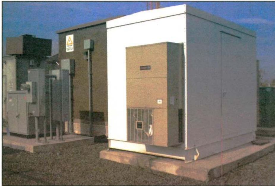
Fig. 5: The building that houses the actual UPS is built around it at a separate facility, then shipped intact to the site by oversize truck.
