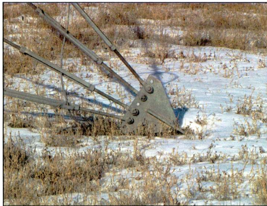
Guy wire anchor steel should be periodically checked below grade for corrosion.
