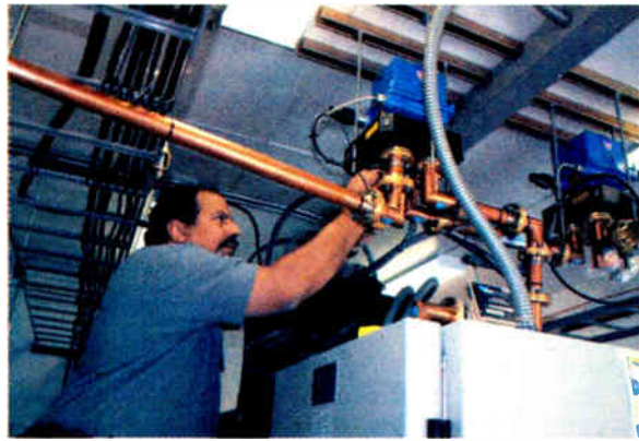
Stu Albert of Albert Engineering Services attaches the rigid transmission line to the coax switches at the new Norsan tower site.
