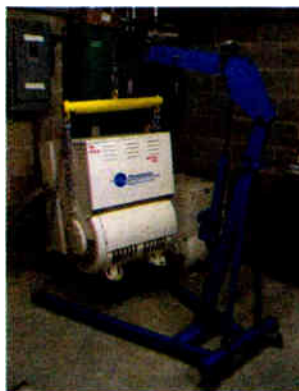
Fig. 3: A sling added to the engine hoist keeps the Phasemaster from tipping as it's moved.
