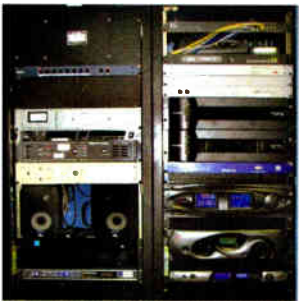
WMMS(FM) transmitter processing racks.
