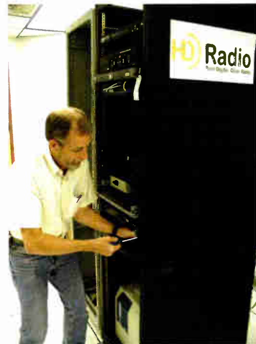
O'Shea with the HD Radio conditional access equipment test rack which holds, from top, a Harris NeuStar processor, Ibiquity test exciter auxiliary unit, Harris Importer, Netgear network switch, NDS Protector and NDS Initiator.
