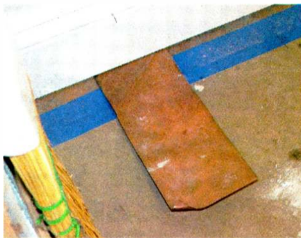
Fig. 1: A copper pigtail for studio grounding
