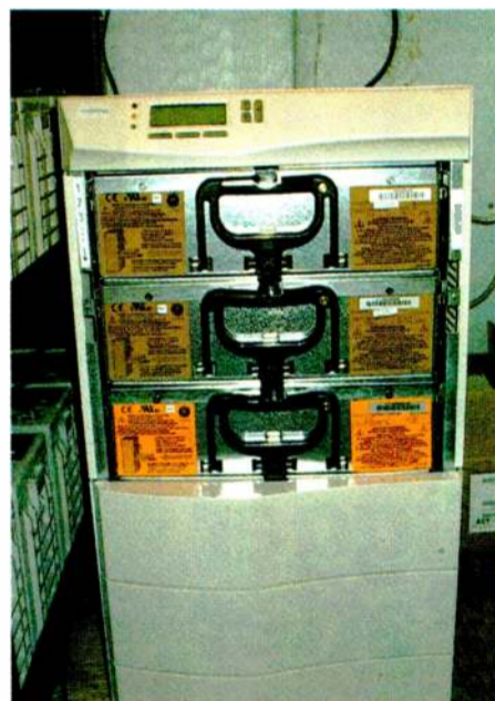
The Bomara inverter/charger with the cover off.
