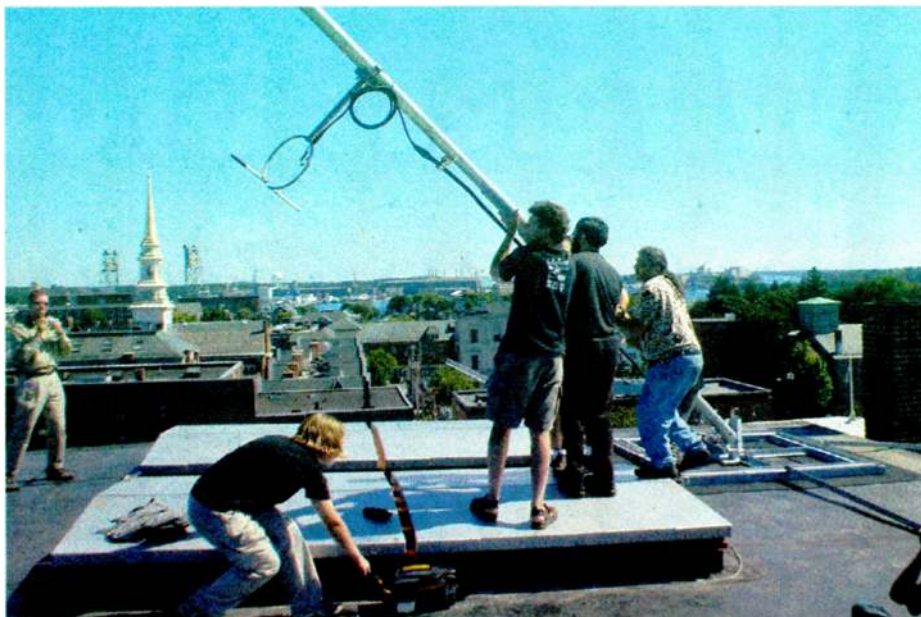
WCSA(LP) in Portsmouth, N.H., installed a custom, freestanding Dielectric Communications DCR-L Dipole antenna rig. Eastern Communications of Saco, Maine, donated its labor to install the antenna, which is mounted on a weighted base.
