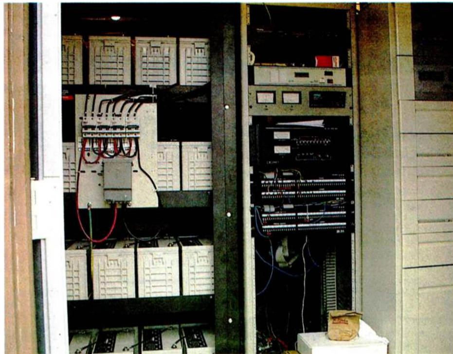
UPS battery power unit, on left, occupies a space where a Sparta tube transmitter had been. The rack next to it holds STL, remote control and backup exciter; the main Harris transmitter is further right.
