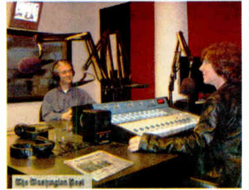
Radio Systems consoles and wiring are in use for Washington Post Radio.
