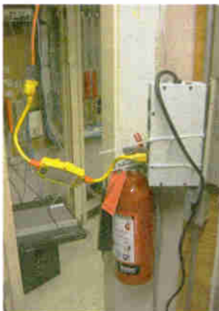
Fig. 3: This temporary lashup of the AC-4 ensures a dry basement.
