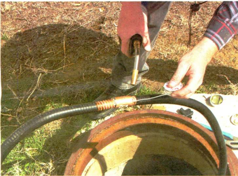
An airtight temporary splice is made using copper strap and tubing to hold things together until a permanent splice can be obtained from the manufacturer.
