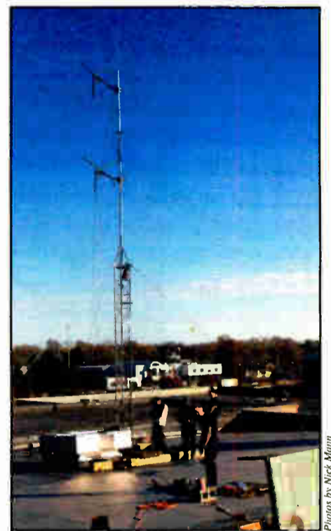
Prometheus Radio volunteers work to secure the tower supporting a Nicom antenna for Radio Free Urbana on the roof of the town post office. WRFU was the ninth 'barnraising,' the term Prometheus uses for building an LPFM.
