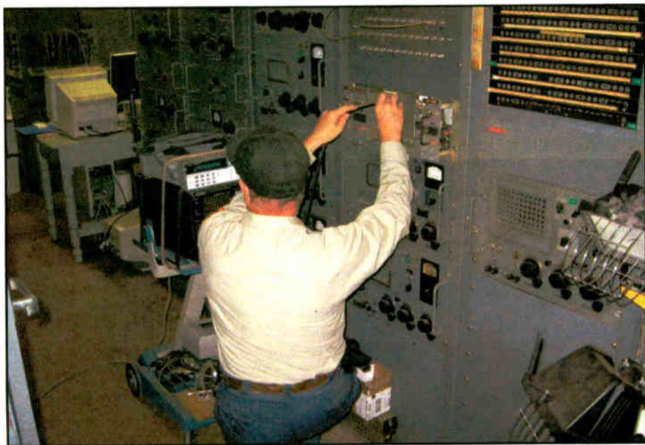
Steve Hawes checks the frequency of an exciter for a PW-15 transmitter.
