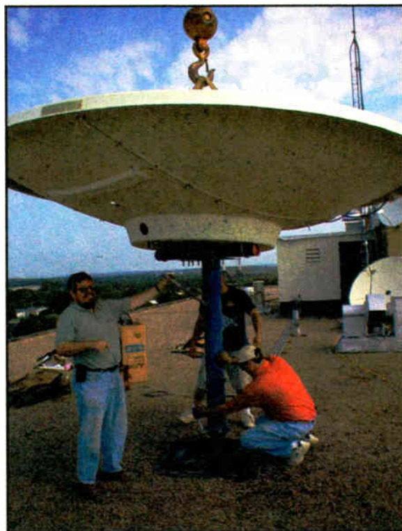
John Huntley, left, and SJT Systems' Scott Tickler tightening support pipe bolts.
