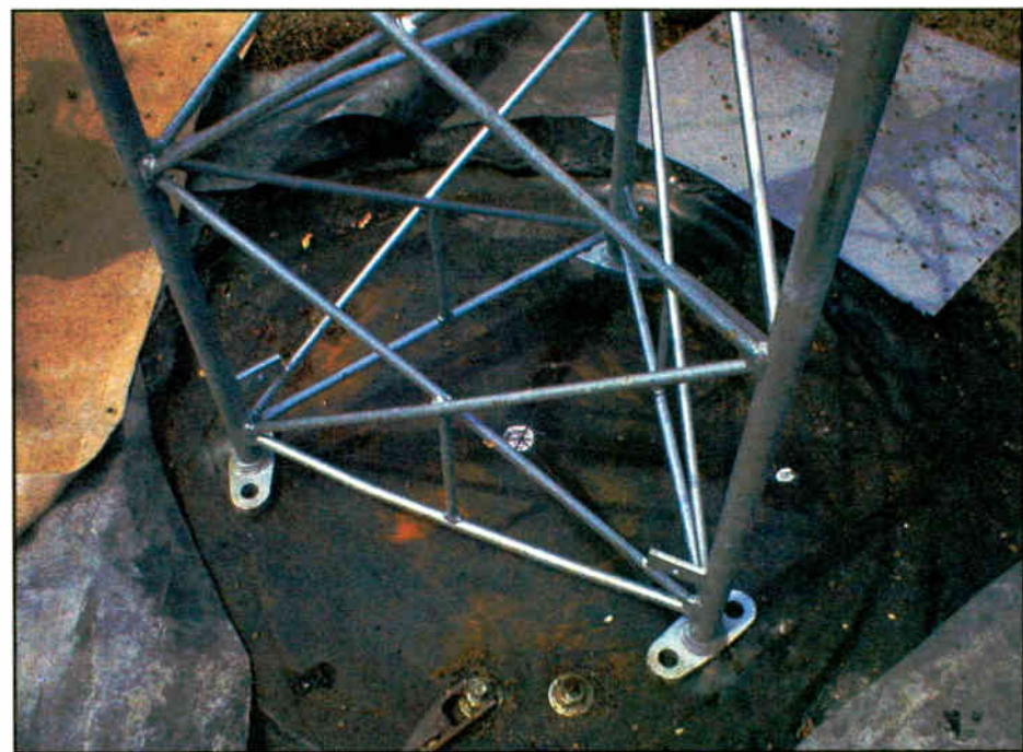
Tower base and plate, with alignment marks visible. A welding ground is attached to the bolt at bottom of picture.
