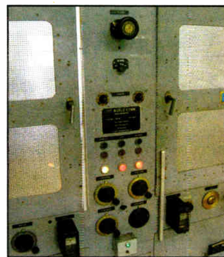
Front panel of 1942 Press Wireless PW-15 transmitter in operation on KSM 12.993 MHz frequency.
